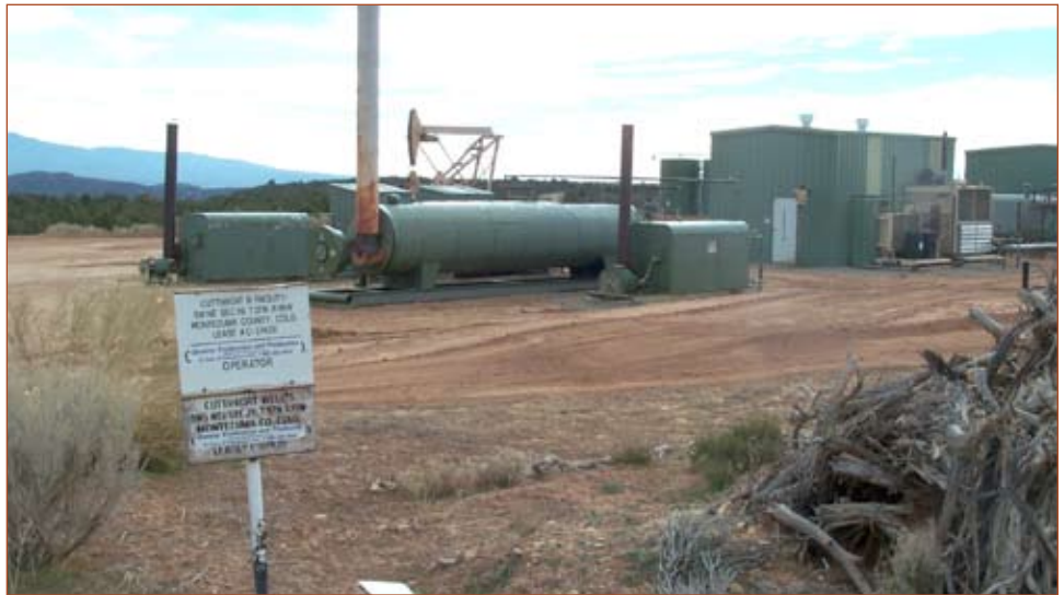
An existing gas well in Canyons of the Ancients, on Mockingbird Mesa.
