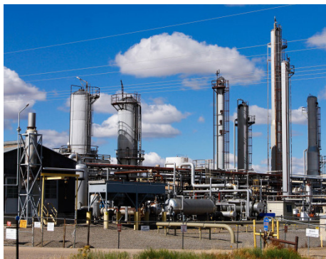
Leakage from natural gas processing facilities is a significant contributor to the methane problem.
